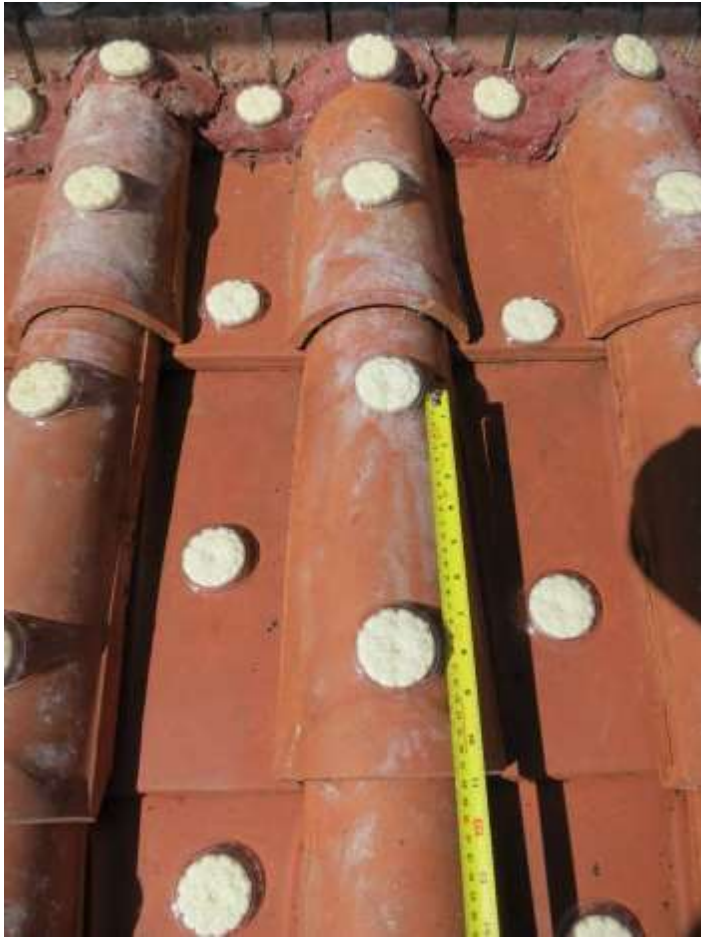
Figure 4. South roof treated with Bird Free .
