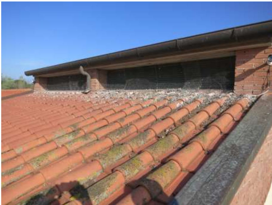
Figure 1. South roof prior to cleaning and treatment.
